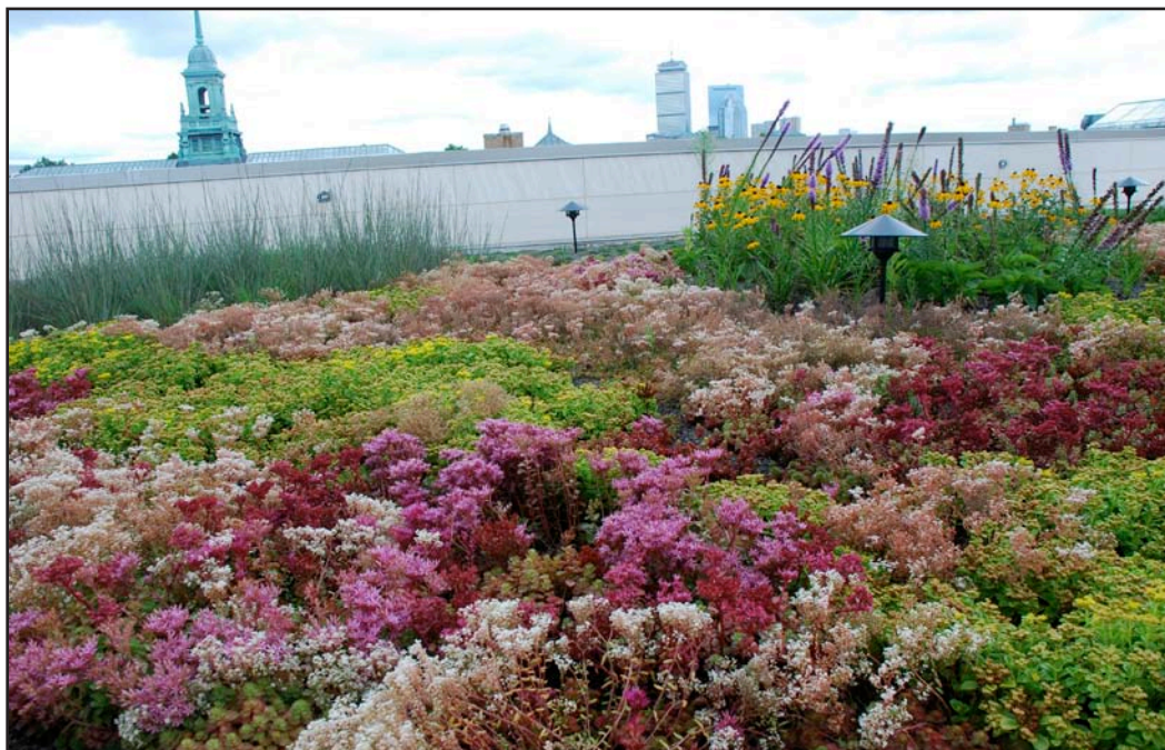
Vegetated green roof at Simmons College, Boston installed by Apex Green Roofs over a Sarnafil PVC membrane
